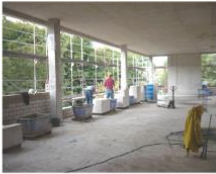
Highly effective insulation
